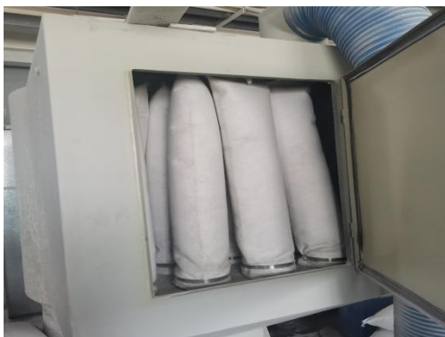
淋砂机废气收集设施
